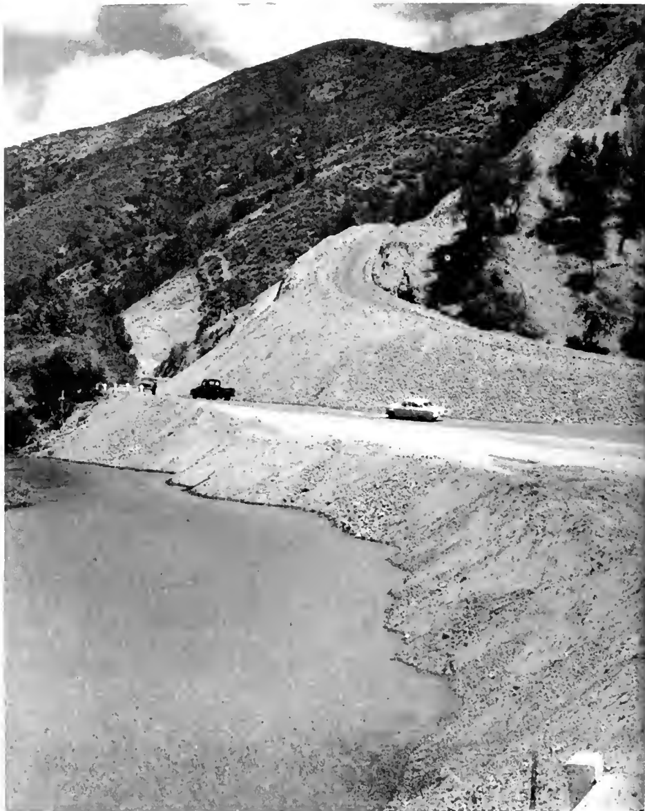
Looking westerly along shores of Laurel Dell Lake in Lake County at the big cuts near westerly end of the Laurel Dell-Tule Lake project. New embankment extends in foreground across small bay of lake.
